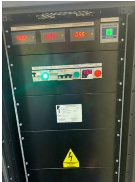
High voltage Power supply
