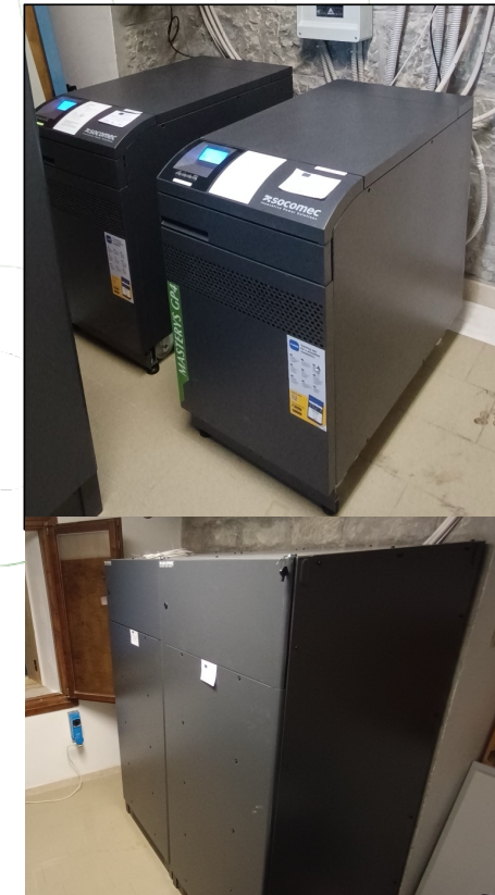
Monte Cimone UPS systems with battery packs
