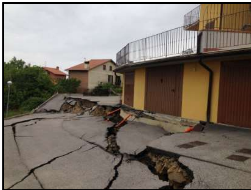
Complex landslides, slides
